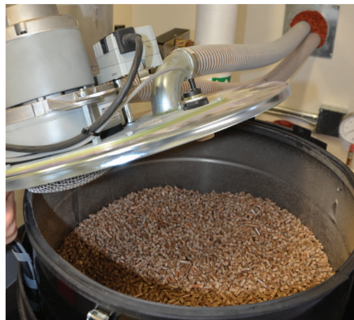
The wood pellets that fuel the boilers are sawmilling byproducts. Only compressed wood is used in the making of the pellets, no bonding agent. They're seen here inside one of the boiler's "day bins."
