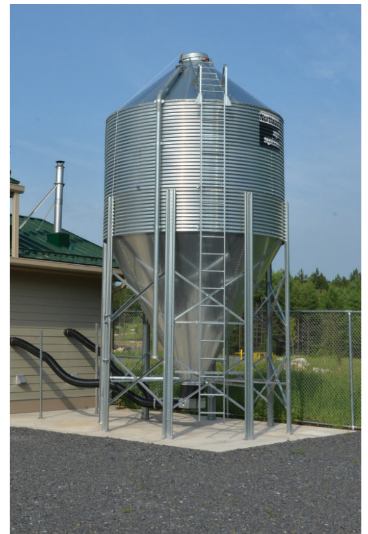
Wood pellets are bulk-delivered to the facility and blown into an outdoor hopper, from which the boilers automatically draw when needed.
