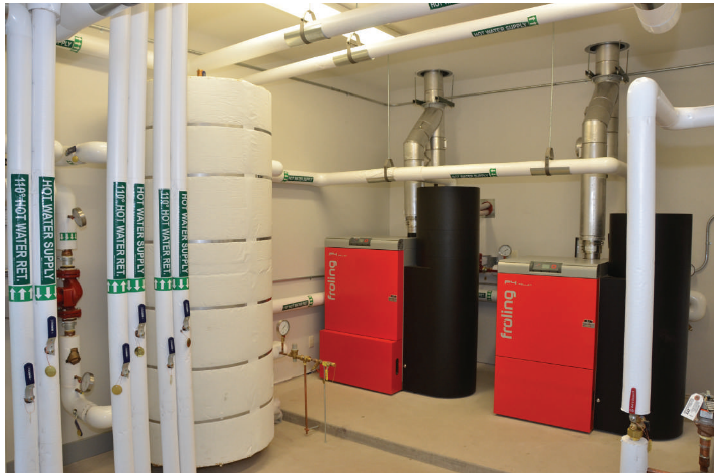
The boilers share a main mechanical room with a super-insulated, 400-gallon buffer tank. All supply and return lines to both buildings run underground.
